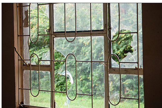
Figure 2. Uraki Secondary School classroom for music with broken windows
